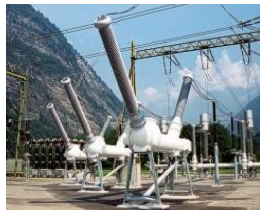
HV Circuit Breakers
