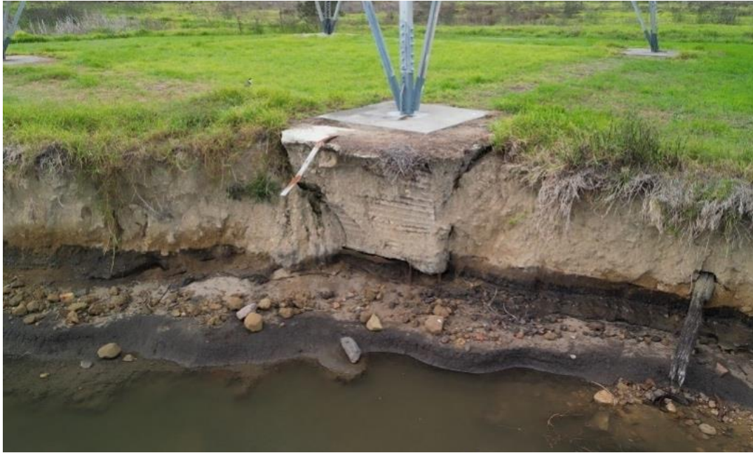
Observed scour at the tower site (Australia)
