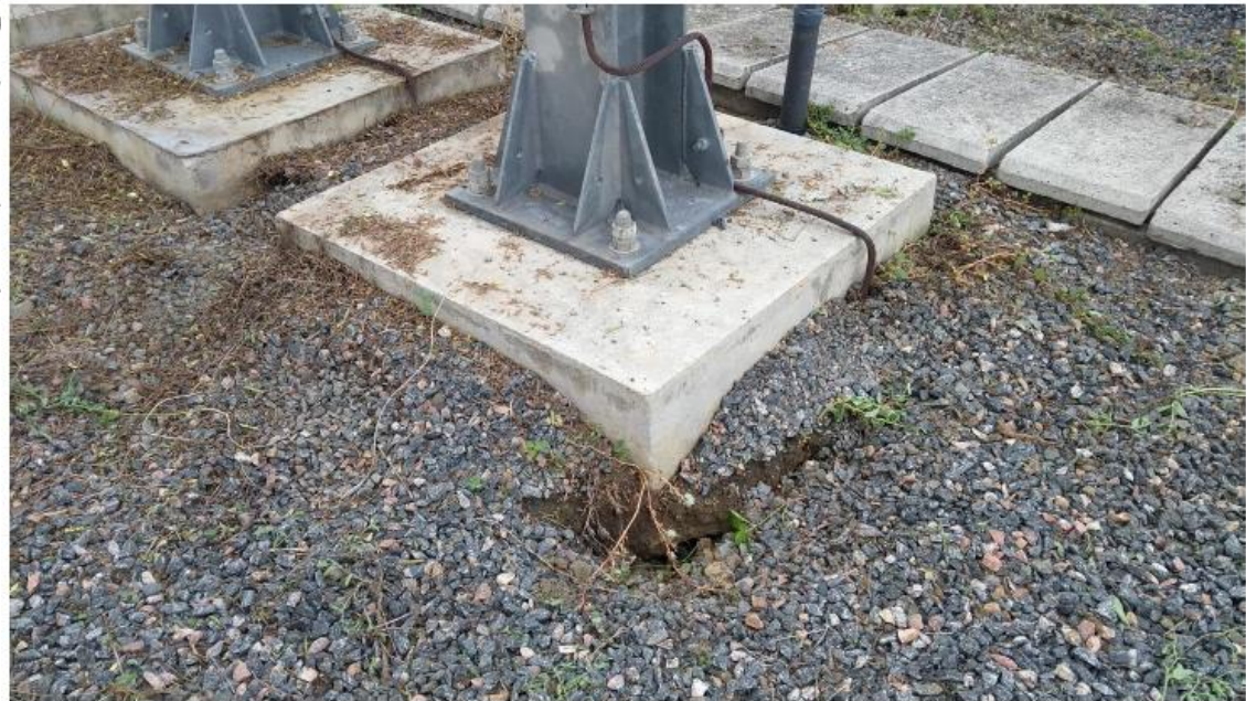
Settlement of landfill near foundations
