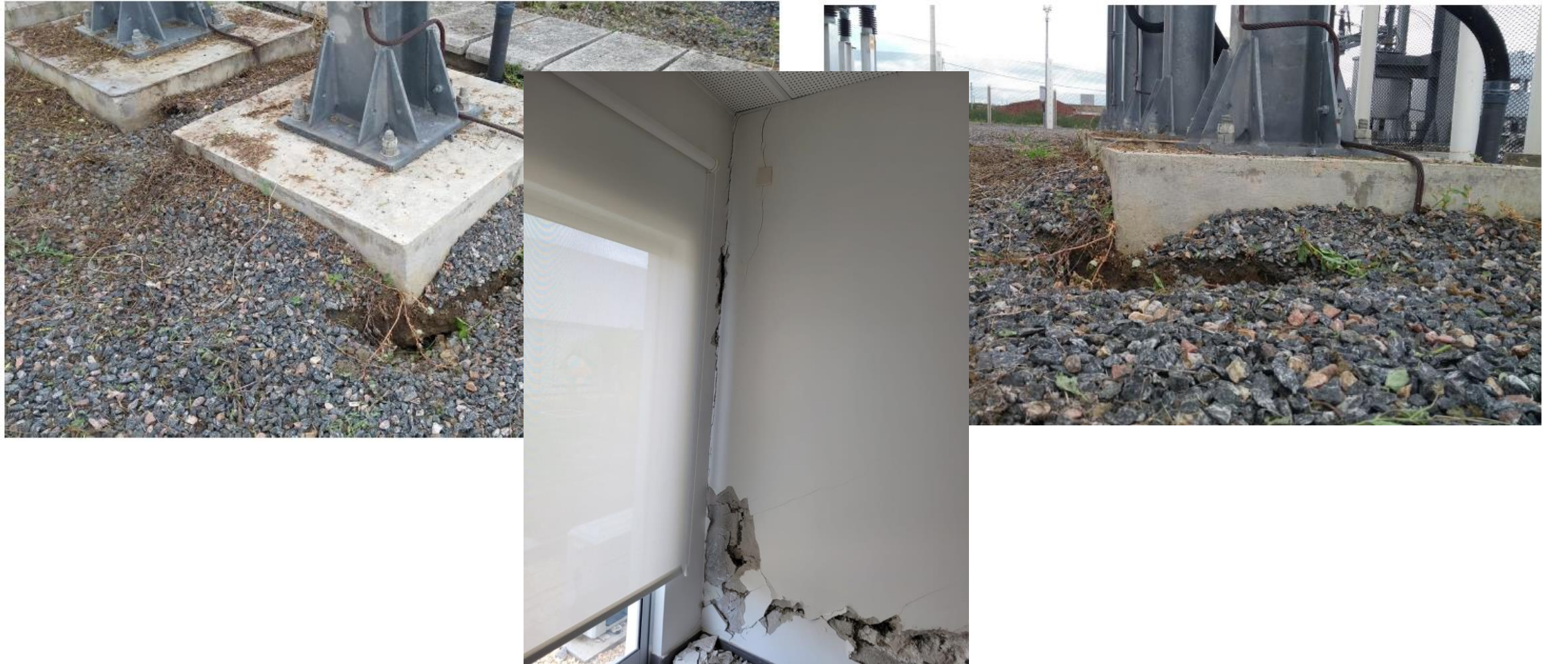
Settlement of landfill near foundations (Brasil)
