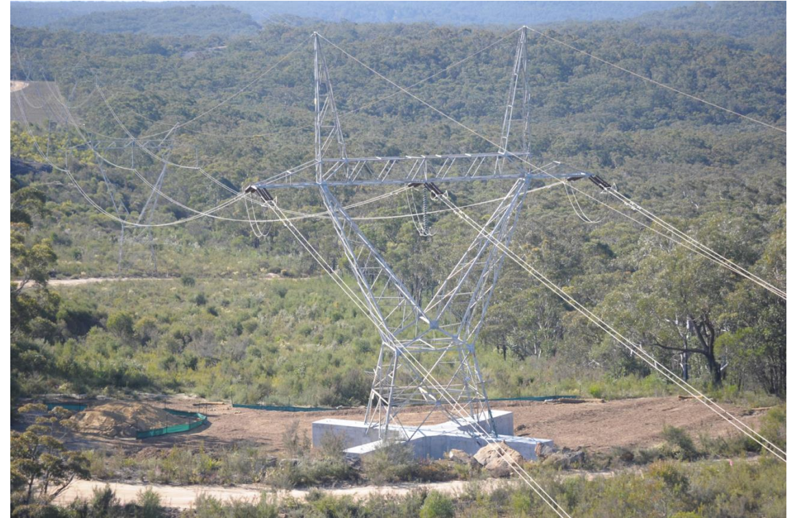
Tension tower with the cruciform tie-beams (Australia)
