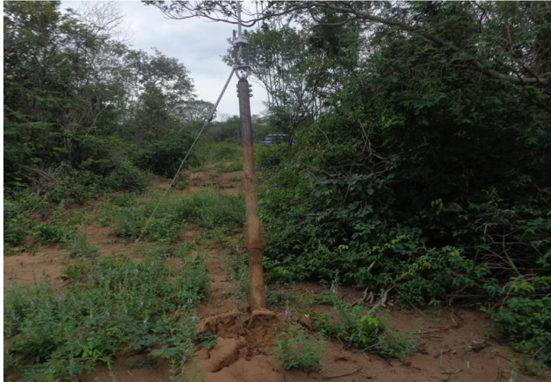
Geotechnical rupture of the helical pile (Brasil)
