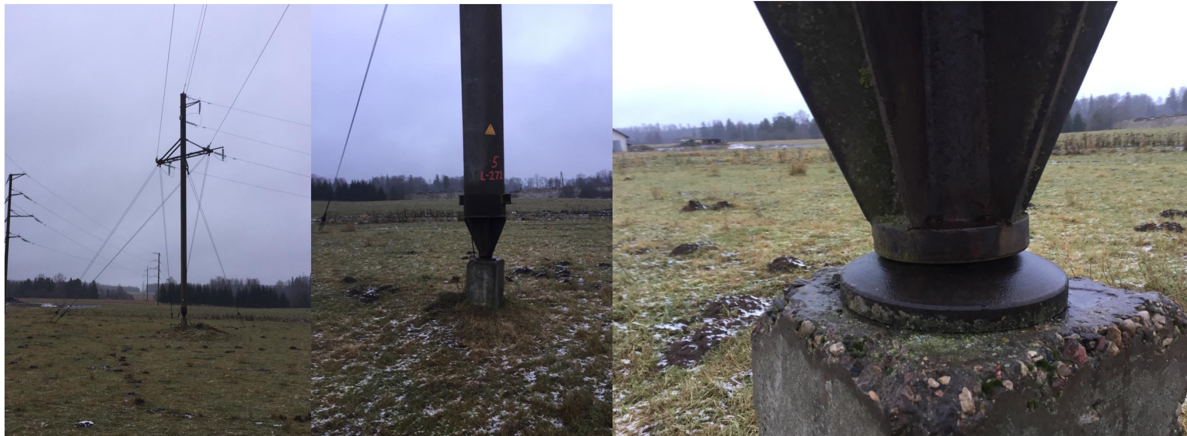
Line 110 kV (Latvia)
