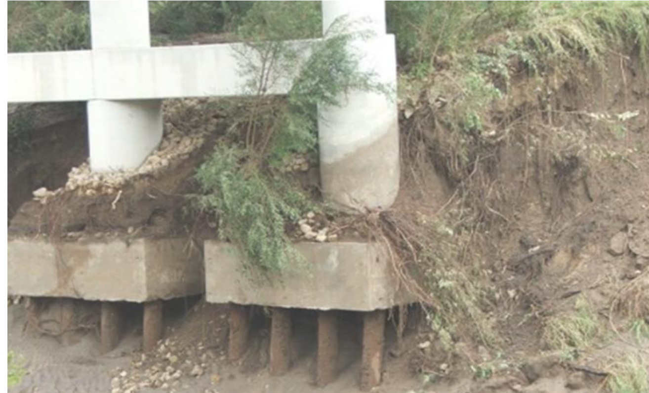
Scour around piled foundation
